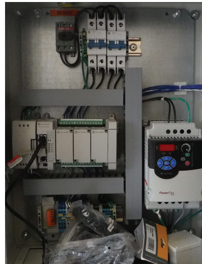
MC3 CONTROL BOX
