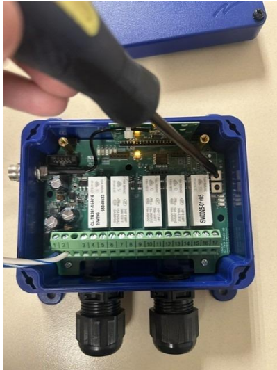
Press FUNCTION to move through relays
